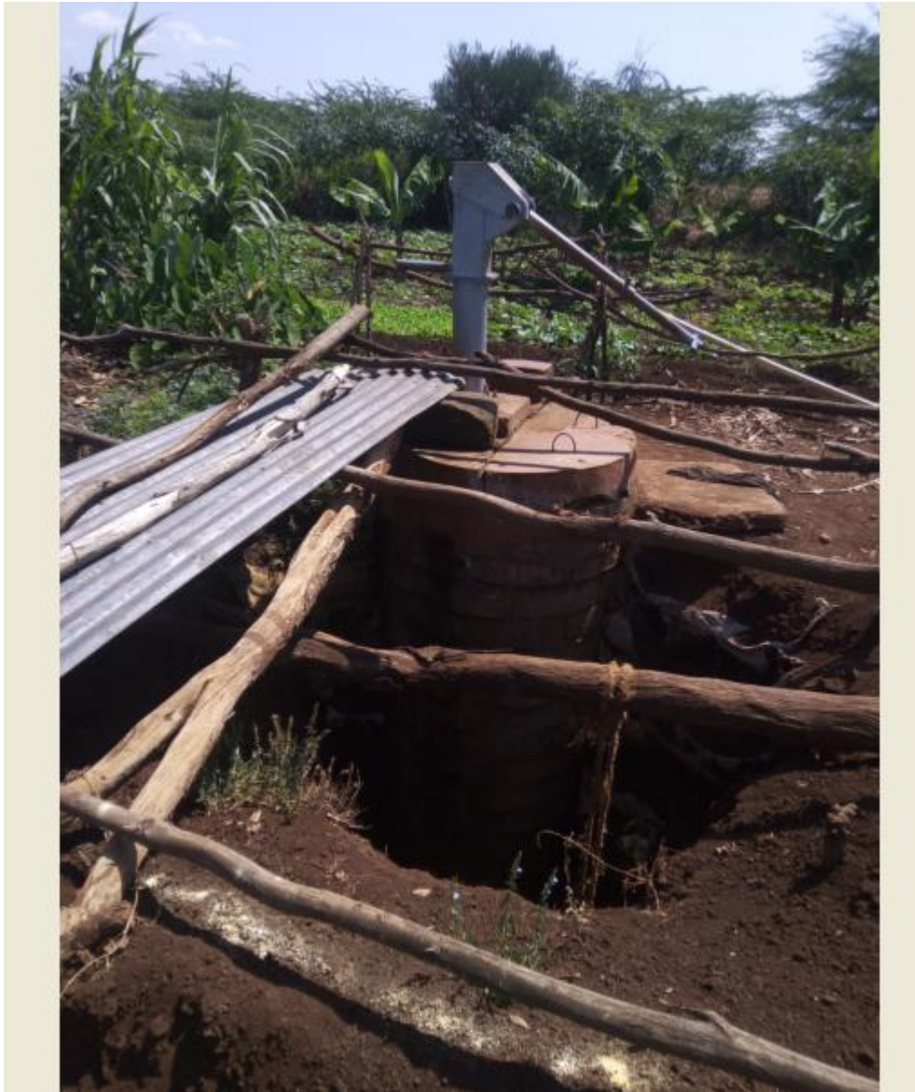
Figure 2: A borehole system (manual hand pumped) and a background of yams, sugarcanes, cassava and beans
